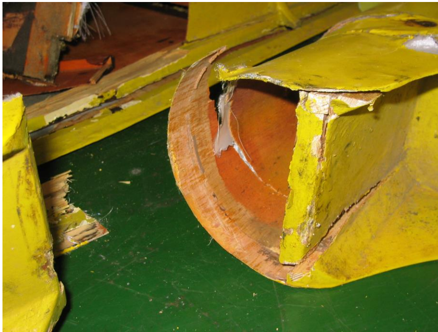
Figure 1 Left elevator D box at Rib No. 1 position illustrating poor glue bond
